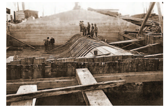
Work crews place steel rebar over wooden forms to create a diversion dam on the Yellowstone River, 1934.
