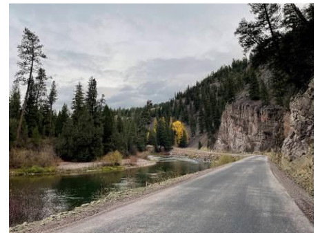
The public can expect temporary delays this month along Johnsrud-McNamara Road as workers chipseal the popular route along the Blackfoot River. (BLM photo by David Abrams)
