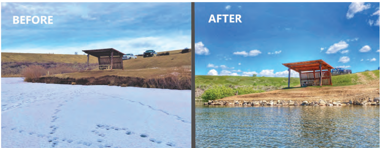
Before and after photos of shoreline improvements at Big Casino Creek Reservoir near Lewistown.
