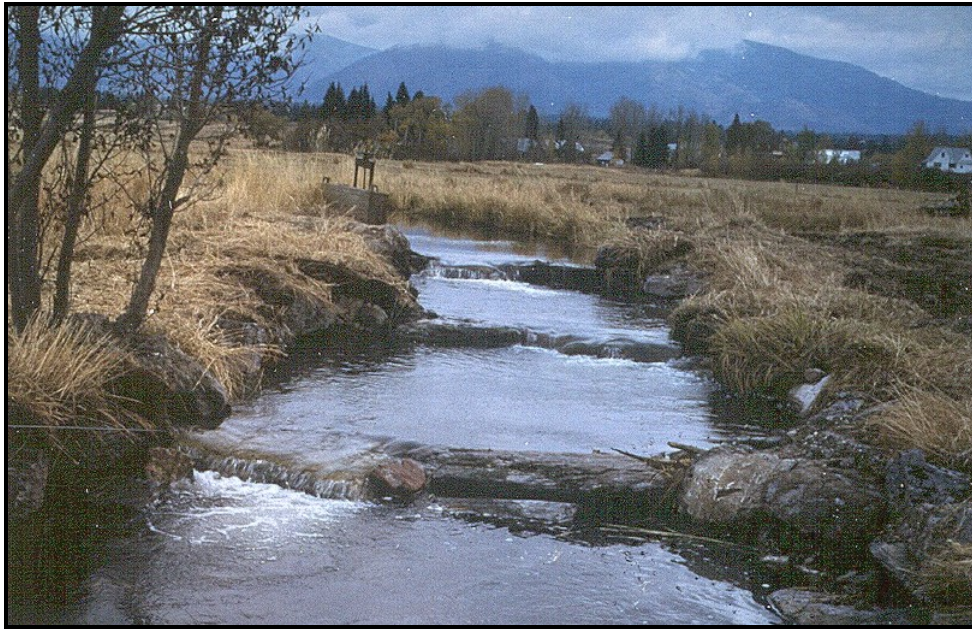
Photo Illustration 2. Installation of a series of step-pool structures in Warren Creek located near the town of Ovando. These step-pools provide for fish passage and create head to deliver water down a water irrigation diversion located on the left side of the photographs. Upper photo shows channel during construction of step-pool structures. Lower photo shows completed step-pool structures following construction.
