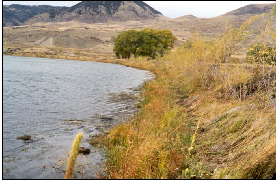
Photo Illustration 3. Restoration of 3,200 feet of eroding river bank on the Missouri River located near the town of Cascade. This project involved bank sloping, placement of salvaged sod, transplanting of approximately 500 willow clumps and the installation of riparian fencing to improve habitat for resident rainbow trout and brown trout. Upper photo shows eroding river bank before restoration. Lower photo shows river bank after restoration.
