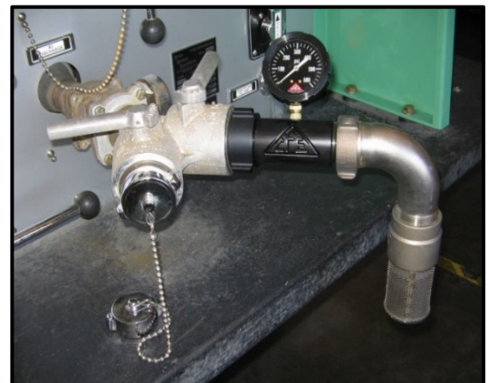
Figure 10. Pressure valve attached to the footvalve.
