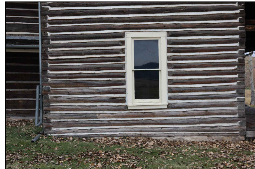
CHIEF'S HOUSE SOUTHWEST CORNER WITH SETTLING
