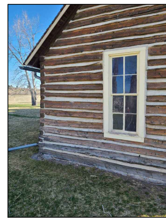
4 DETERIORATED WINDOW SILL ON WEST FACE A5
